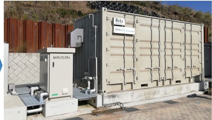
25kW Test System
